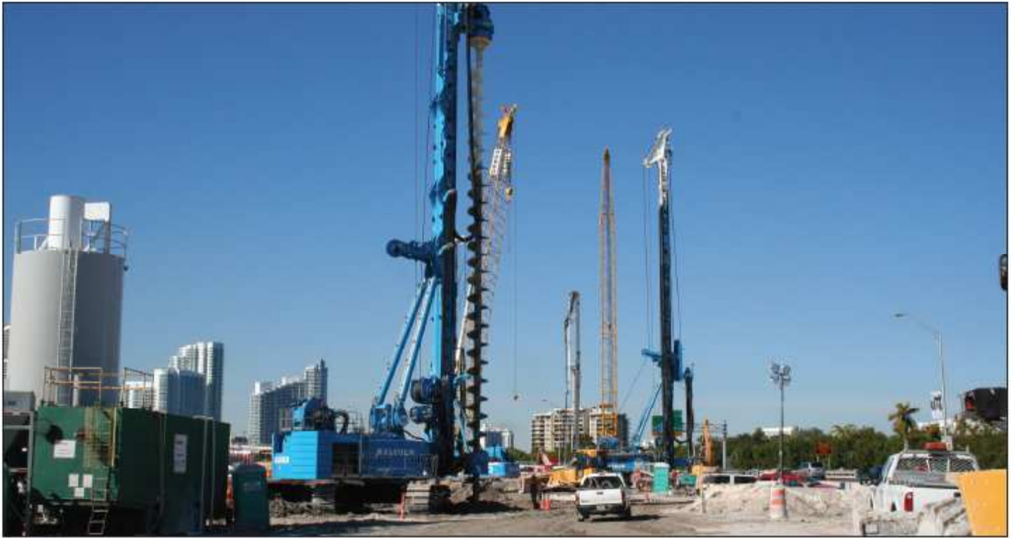
Malcolm Drilling is installing a support of excavation by creating the break-in plug on Watson Island to provide a non-permeable block for the 43 ft. (13.1 m) Tunnel Boring Machine.
