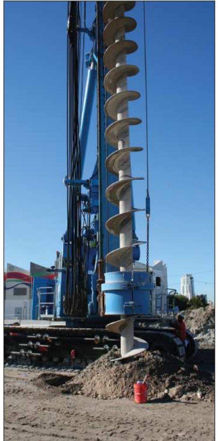
A BAUER BG 50 with a continuous flight auger pre-drills 48 inch (1200 mm) shafts.
