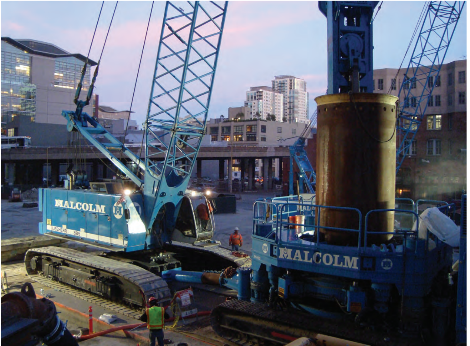
Front cover: Oscillator Installation, San Francisco, CA Back cover: Rotator Installation, San Francisco, CA
