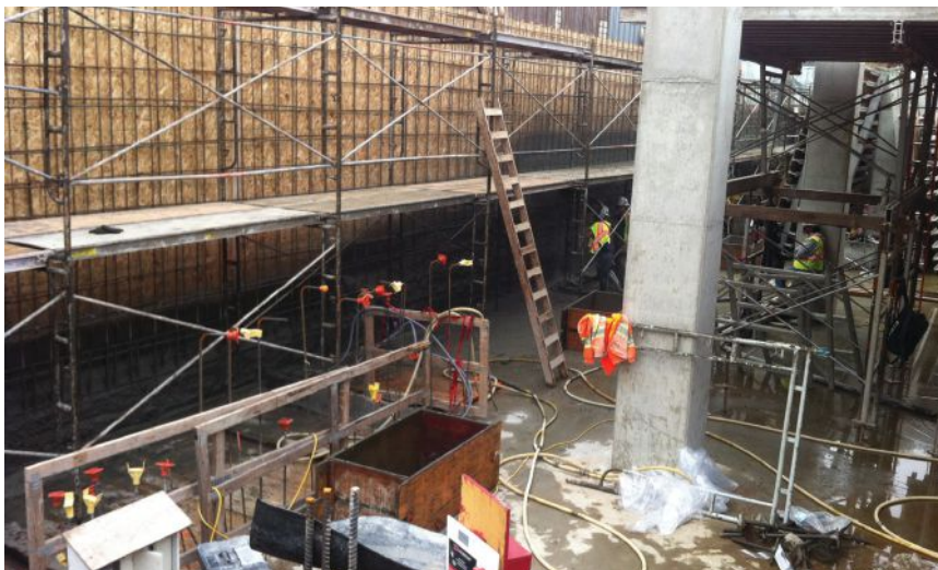
Xypex was used to waterproof the foundation of Vancouver’s new Neelu Bachra Centre.
