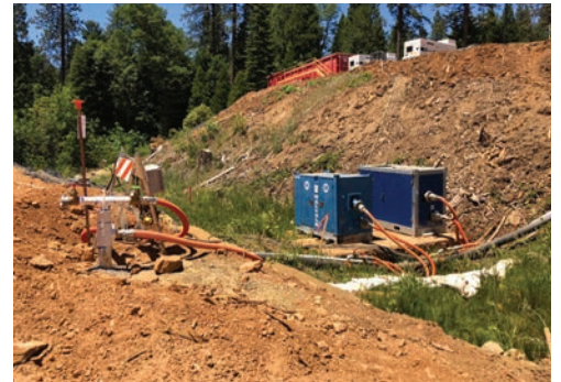
BOTTOM RIGHT: Dual HDPE discharge header pipe used to convey the dewatering water from the wells to the discharge location. The header pipe was split to reduce the TDH allowing more water to be pumped from the wells.
