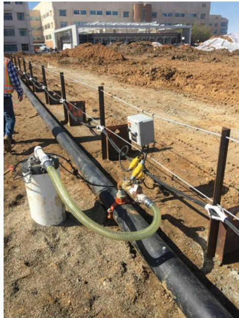
OPPOSITE: Interior deep wells located along the inside perimeter of this cutoff shored excavation that extends 50 feet deep.
