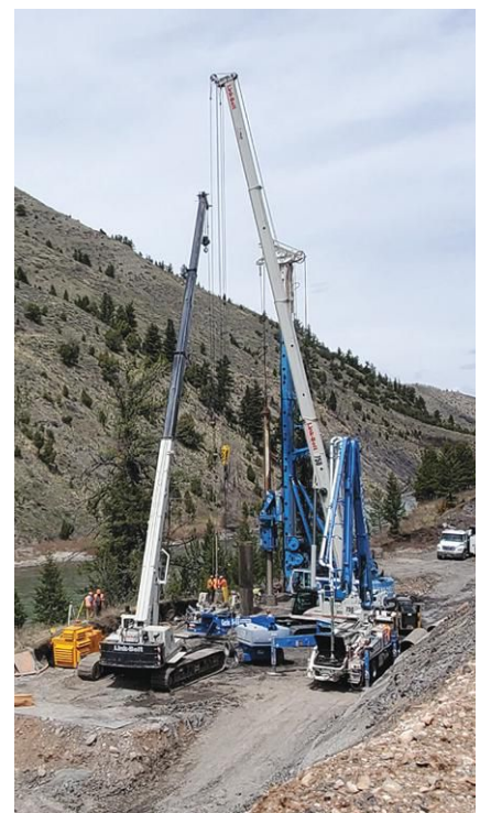
Drilled shafts installed by Malcolm Drilling are part of the Wyoming Dept. of Transportation's plan to improve Highway 191 and add a bicycle path.
