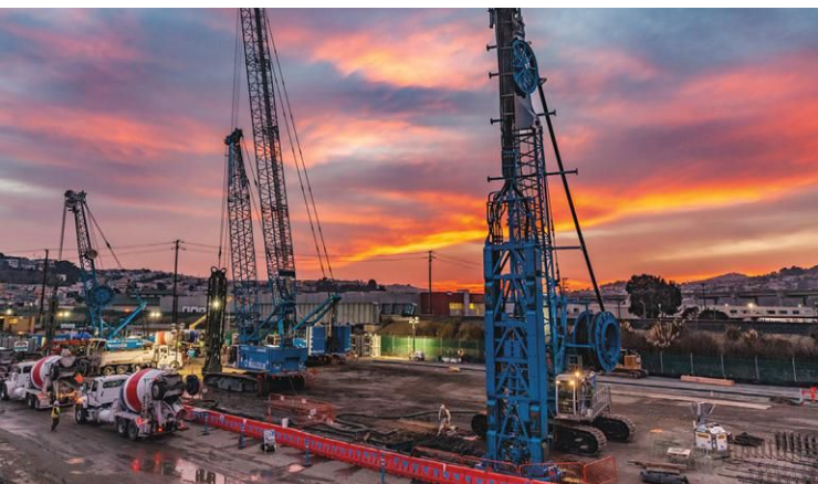
Malcolm Drilling masterminded multiple tasks simultaneously for San Francisco's Southeast Treatment Plant replacements.
