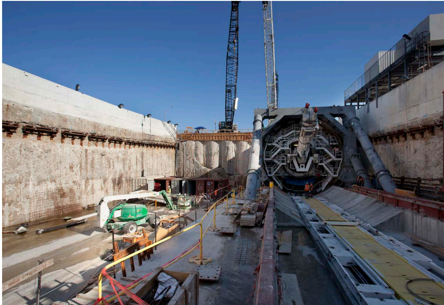
ABOVE: Anchored CSM wall, Miami, FL BELOW: CSM shaft, Fremont, CA OPPOSITE: CSM equipment, San Carlos, CA
