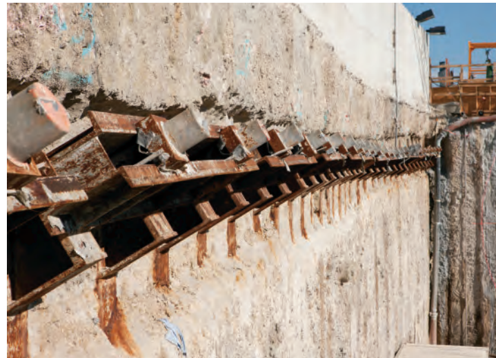
CSM wall with tieback anchors (photo by Mike Butler and Dan Riebe)
