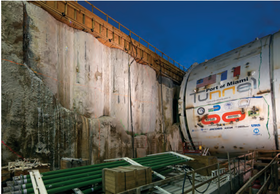
Tunnel boring machine at the entry plug (photo by Mike Butler and Dan Riebe)
