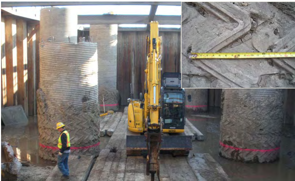
Figure 13 Exposed Texture on the Drilled Shaft Surface, Huey P. Long Bridge
