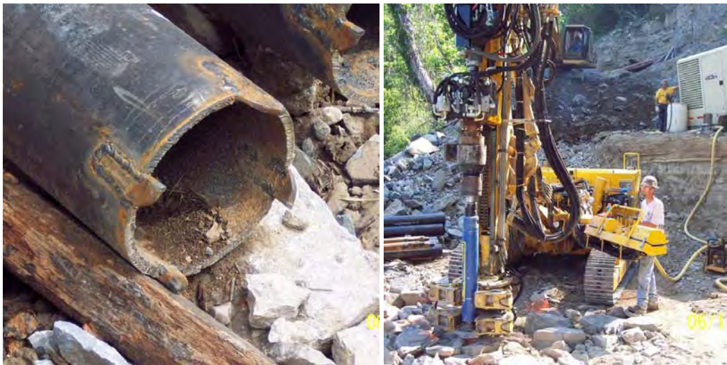
Figure 3 Micropiles Cased Through Boulder Fill for the Cumberland River Pedestrian Bridge, Nashville, TN
