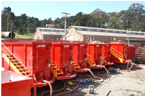
Figure 17: Slurry Tank Battery
