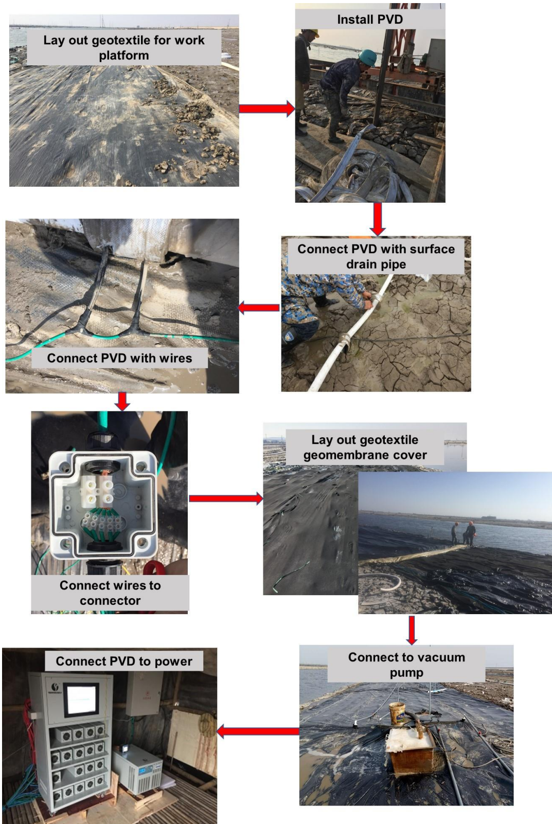
Figure 10. Procedure of installation and construction (courtesy of Hangzhou Shenyuan Environmental Sci-Tech Co. Ltd).
