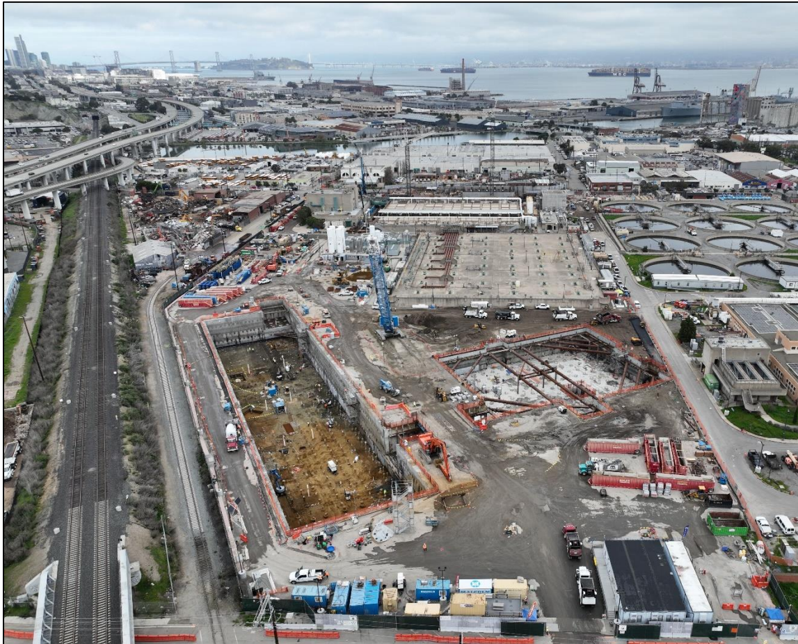
Fig. 17. Overview of project site with completed diaphragm wall excavation at Facility 610 (left) and internally braced CSM shoring wall at Facility 600 (right)
