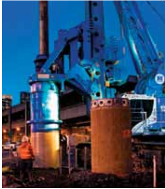
Crews install the launch pit to prepare for the world's largest TBM.
