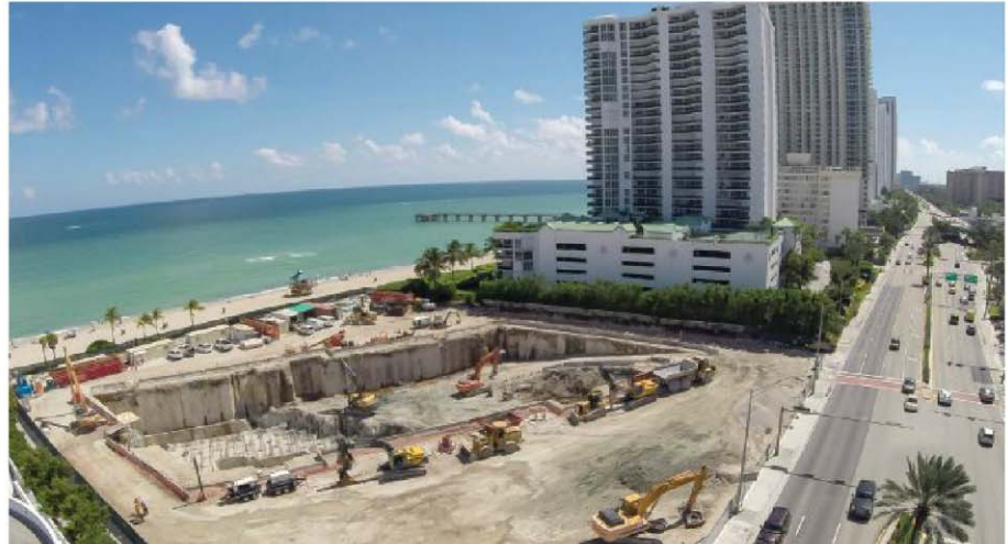
For the foundation of the Jade Signature tower in Miami, Malcolm Drilling avoided sealing and dewatering challenges by installing large diameter soil mixed piles.
