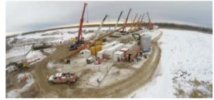
Michels completed a 7,200-ft HDD under the Athabasca River in Alberta, Canada.
