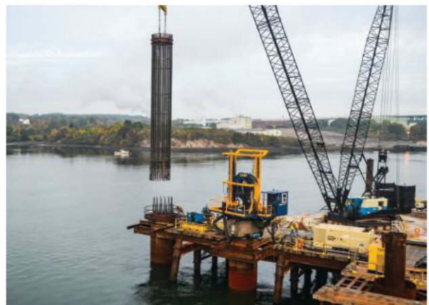
Case Foundation constructed drilled shafts for the bridge replacement between New Hampshire and Maine across the Piscataqua River.
