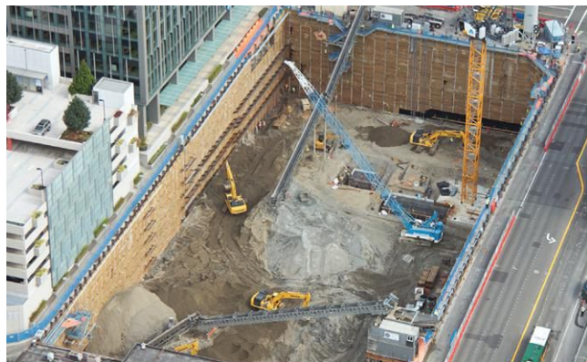
Malcolm Drilling helped to design and install an elaborate water system in this temporary shoring pit during construction of a future high-rise in Bellevue, Wash.
