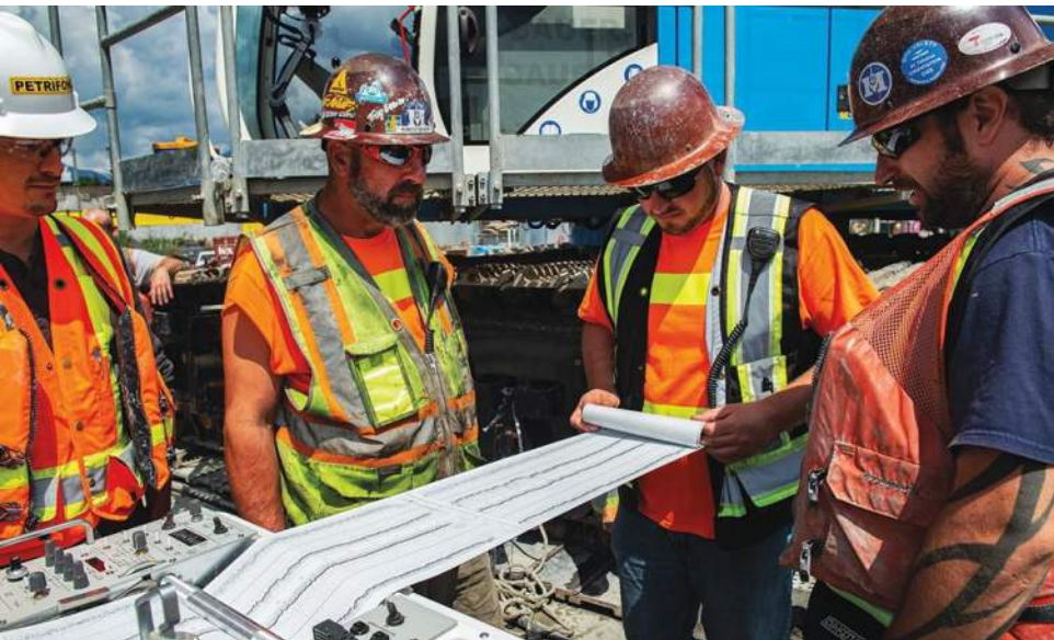
Malcolm checked the verticality of the slurry wall with a Koden ultrasonic drilling monitor.
