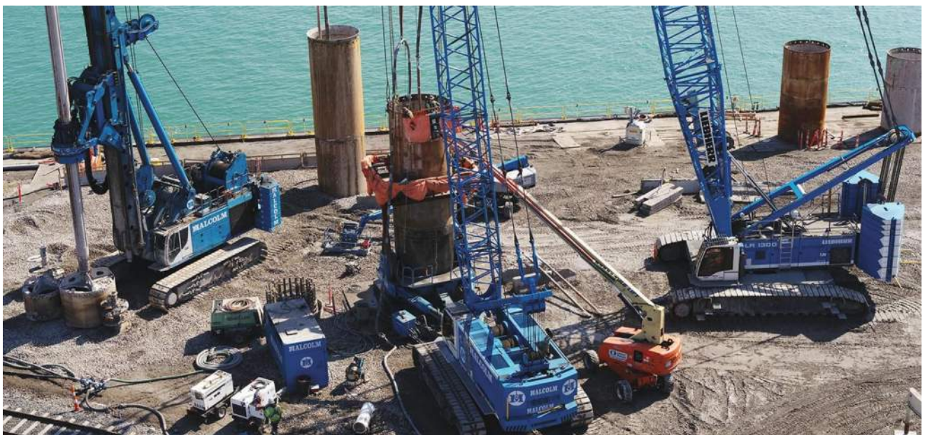
Using its BG50 drilling machine fitted with custom-made drill tools, Malcolm drilled through various geological soils to reach hard limestone rock.
