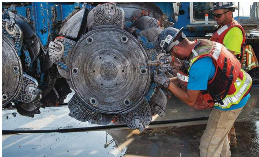
Malcolm used a hydrocutter to cut a 4-ft-wide trench for the slurry walls of the north shaft for the Second Narrows Water Supply Tunnel project currently underway in Canada.
