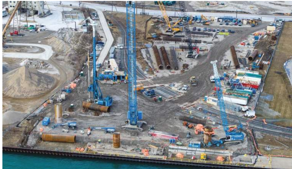
Construction proceeds on the Detroit side of the Gordie Howe International Bridge, the new border crossing between Michigan and Ontario, Canada. Malcolm installed shafts for the main structural support tower and the back span/anchor piers.
