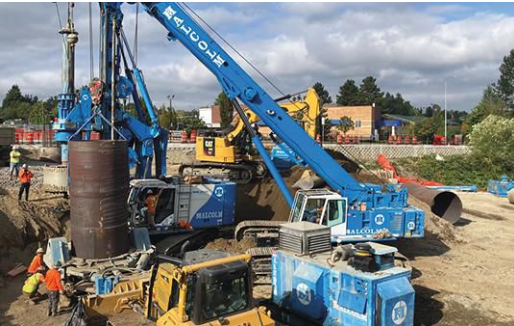
Drilling the 72-ft-deep drilled shafts was done with a BG24 top-drive drill rig equipped with a low-headroom mast, oscillator and 75-ton crane with boom limiter.
